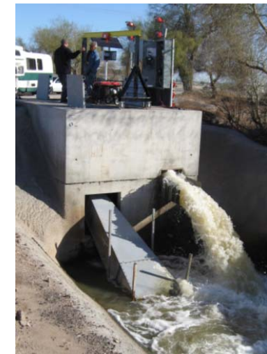
Figure 2: South view of engine-generator foils and vault and draft tube
